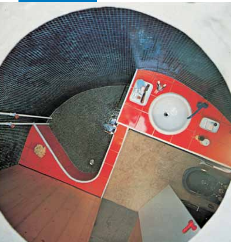
Waterproofed bath-tub and shower
