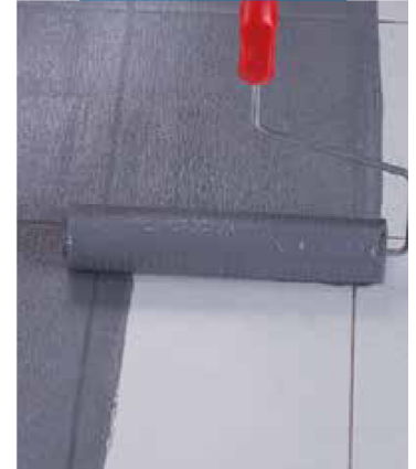
Application of Eco Prim Grip Plus by roller on existing porcelain tiles
